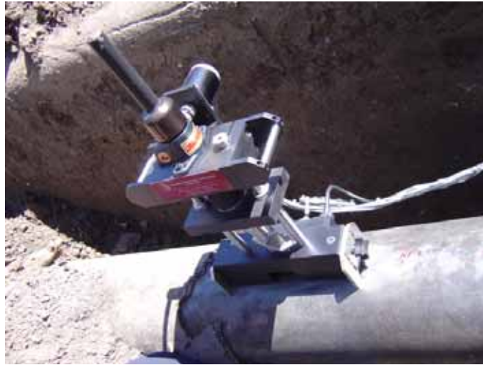
Fig. 1 The testing head of the SSM system is mounted on a 254-mm diameter gas pipeline using DC electric magnets.
