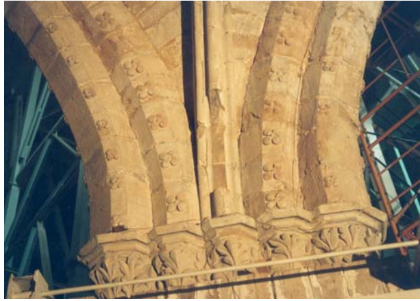
Figure 1: Pier of Tarazona Cathedral affected by damage in compression
