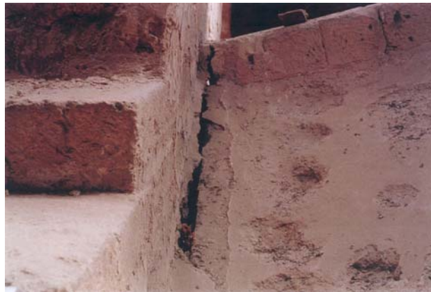
Figure 2: Crack between transverse arch and cross vault in the nave of Mallorca Cathedral
